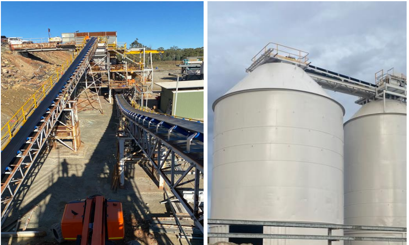
Figure 6: Refurbished conveyor belts at the comminution circuit (left) and the refurbished fine ore bins (right).
