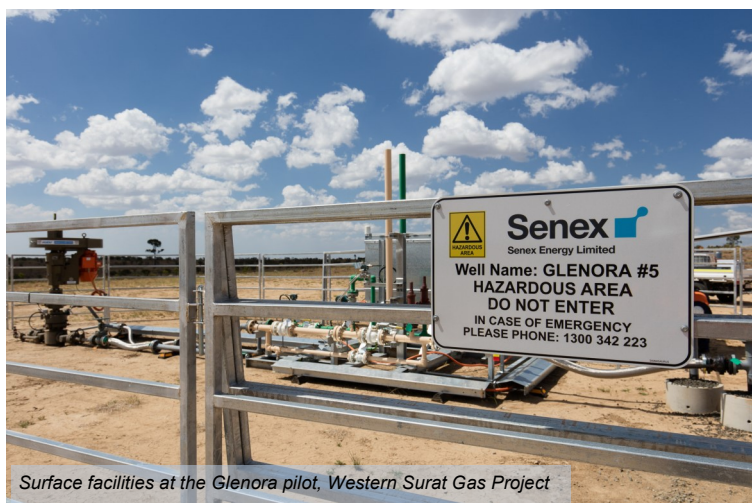
Produced gas at the Glenora pilot, Western Surat Gas Project
