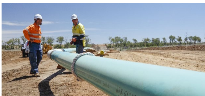
Roma North pipeline
