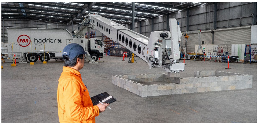
Next-generation Hadrian X ® (H03), operated by tablet, laying blocks utilising new lay-path vectoring protocol
