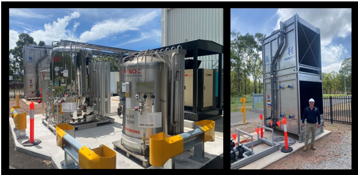
Support infrastructure for the synthetic sapphire growth units installed. Inert gas utilities (LHS) and water cooling tower (RHS)
