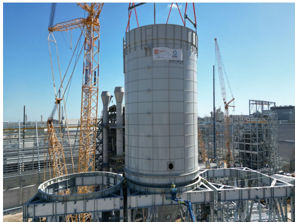
Silo tanks A and B being installed into their frames during Q1 2024
