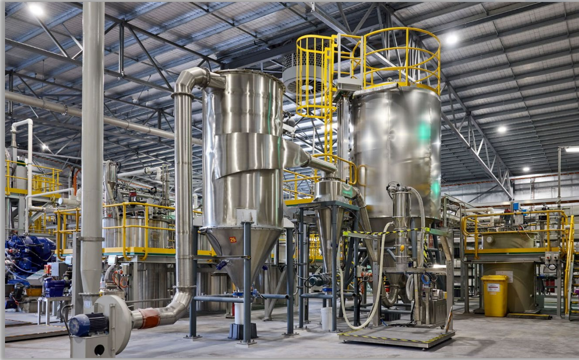
Stage 1 spray dryer under commissioning used for final processing of high purity alumina hydrate
