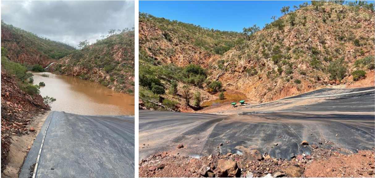
Completion of surface water diversion infrastructure at Capricorn Copper; full following rainfall (LHS) and subsequently pumped dry (RHS).
